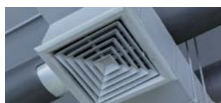
Ventilation duct monitoring
